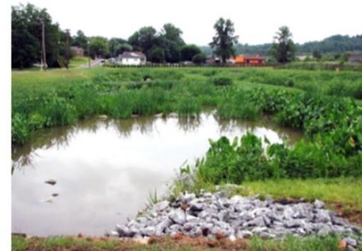
Figure 19. Adding features and topsoil in a large wetland. Side-slopes have already been prepped, and grass is coming up (top). After 1 year, vegetation is successfully established (bottom).
