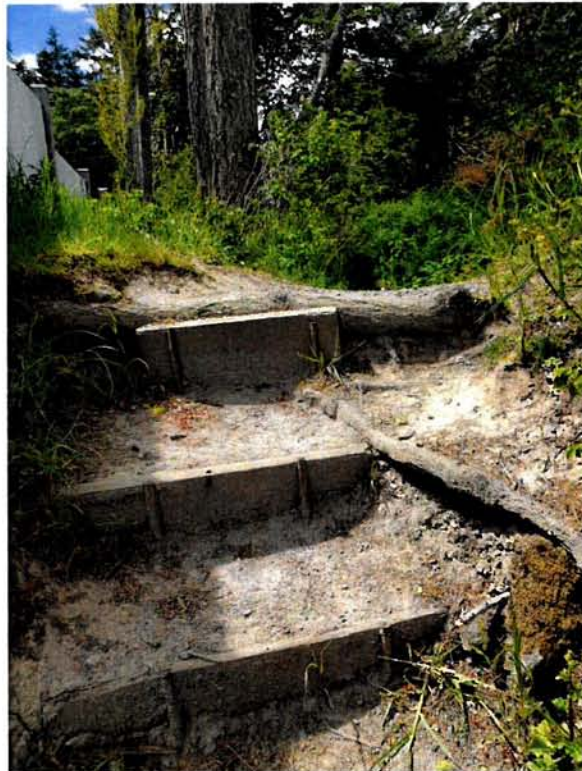
Top. The top of the stairs is constrained by some large tree roots.
