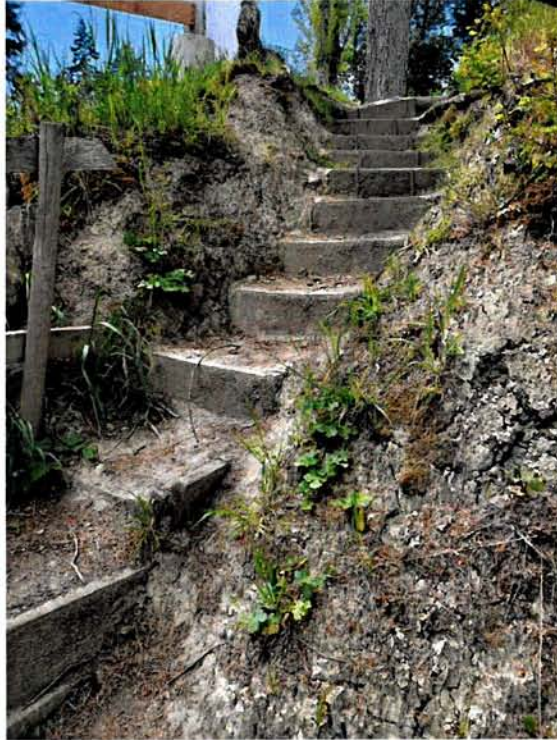
Upper section. The upper section of stairs is constructed of wooden planks well anchored into the soil with rebar. Although the steps are steeper than standard, these are in relatively good condition.
