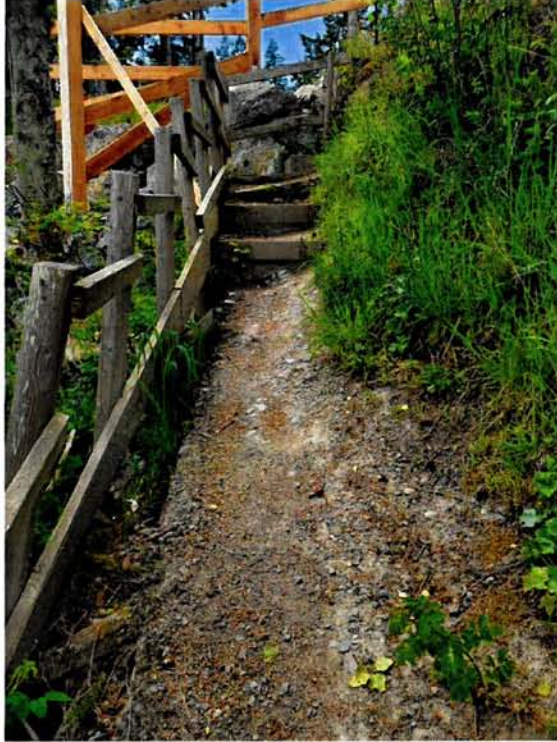
The lower section of stairs is insecure, as is the handrail.
