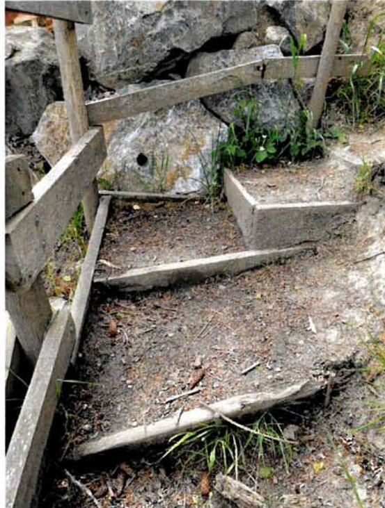
Corner. Halfway up the slope, the stairs make a 90 degree bend. The side facing the beach is poorly supported.
